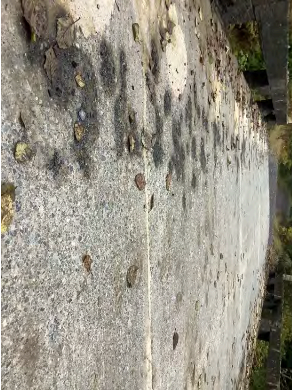
Deck - damage from excavator walking on deck
